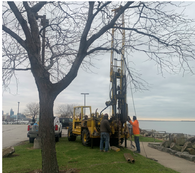
Investigation of subsurface soils for the design of shore protection and dredge containment structures.
