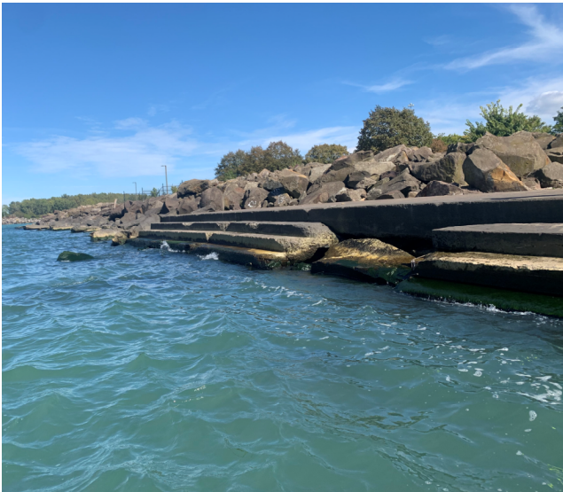
Inspections of coastal infrastructure that will be incorporated or affected by the CHEERS project.
