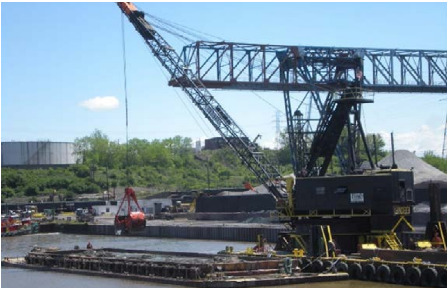
FIGURE 20. A CRANE WITH A CLAMSHELL DREDGE PLACING MATERIAL IN A DREDGE SCOW.
